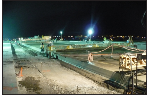
Placement of 18" PCC pavement was constructed at night to minimize operational impacts to airport traffic.
