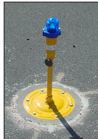
LED lights installed during this project relieve energy demand, reducing the airport's carbon footprint and operating expense.
