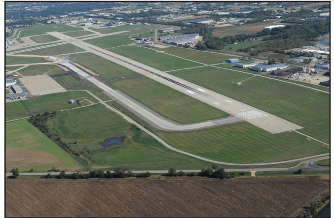
Overall project view looking NE, showing both phases of the project. Phase I (southern portion) is in the foreground and Phase II (northern portion) is in the distance and under construction.
