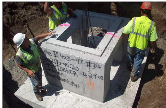
Due to the location of the project in relation to the Missouri River Levee, the drainage structures were designed with wide and deep bases to counteract uplift and to meet ACOE requirements.
